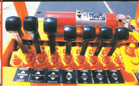
Direct Connected Control Handles
